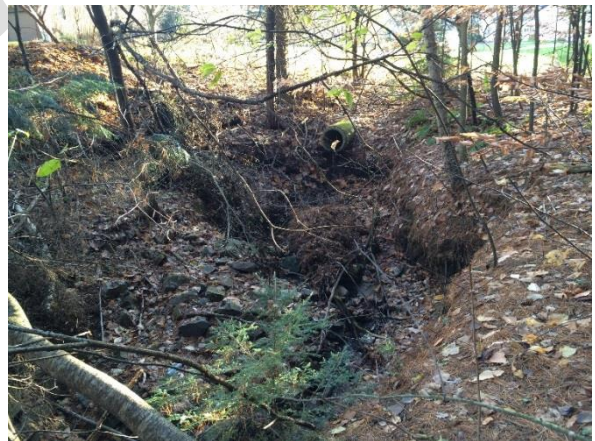
Figure 2: North outfall shows evidence of significantly erosion.
